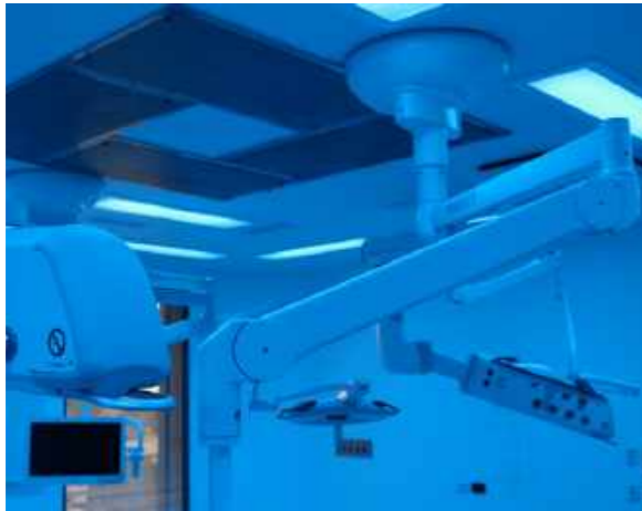
Eagle Lighting Australia supplied Werribee Mercy Hospital with customised Cleanroom CR65L luminaires for use in numerous operating theatres. Controlled by a wall panel, each fitting contained green, blue and CRI90+ white LEDs.
